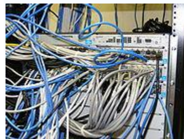
A rack-mounted switch with network cables
